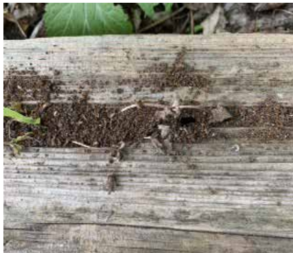
ANT DAMAGE ON WOOD
