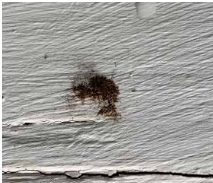
DRY ROT ON HOUSE
